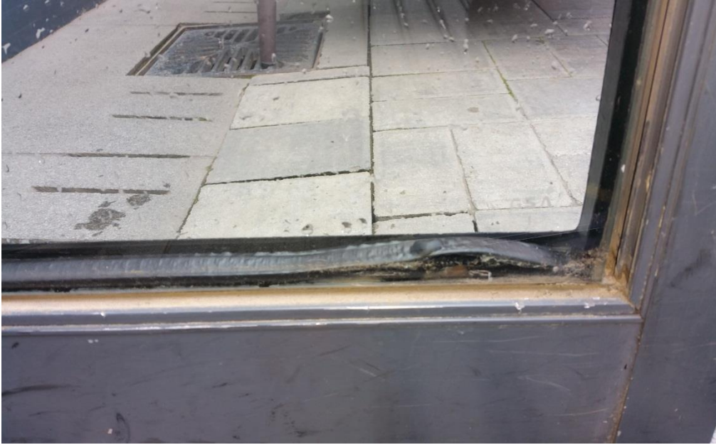
Figure 4: Glass resting on metal frame, due to incorrect setting blocks
